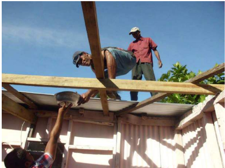
FRIEND Carpenter Setareki Colati leads work on the roofing of a cyclone damaged house
