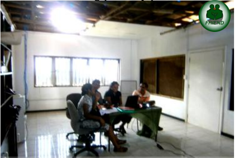
Under a broken roof
